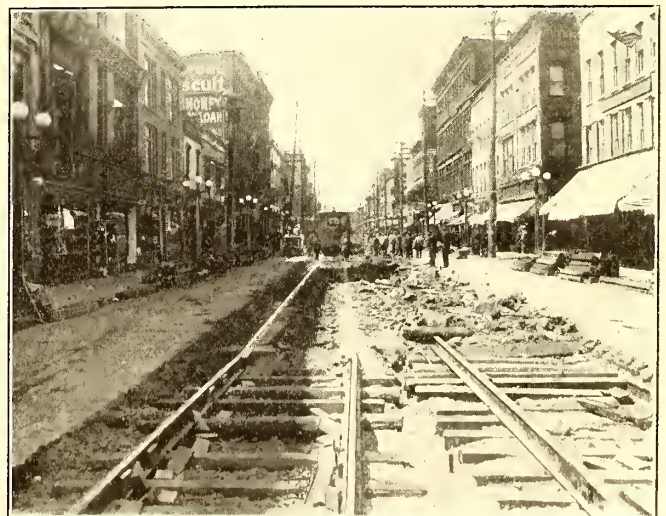
ELMIRA TRACK RECONSTRUCTION—FIG. 7—CONDITION AFTER REMOVAL OF RAILS AND TIES FROM ONE TRACK
